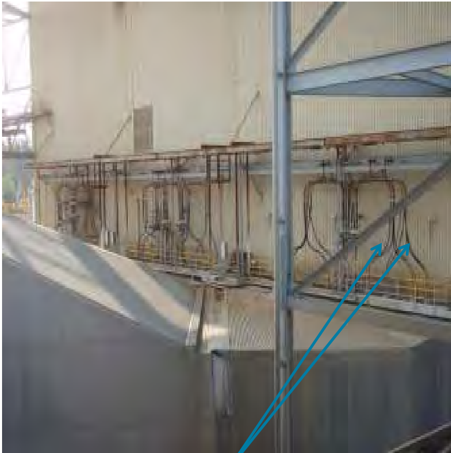
AH outlet injection with 2 parallel injection locations staggered, A&B, 24 lances each
