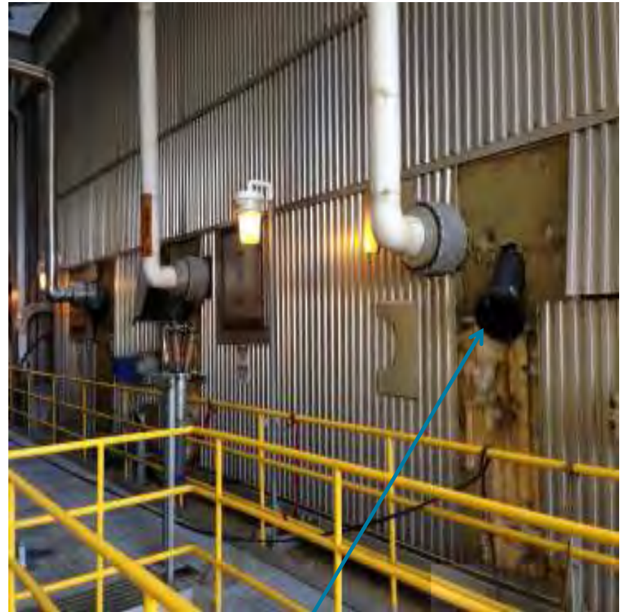
SCR inlet injection utilizing the Delta Wing mixers for ammonia/Nox mixing, 4 lances/box
